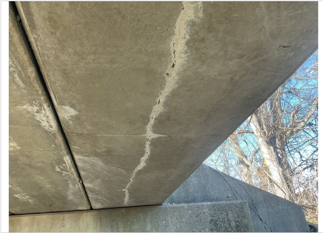
CRACK IN BOTTOM OF BOX BEAM "A", SPAN #1
