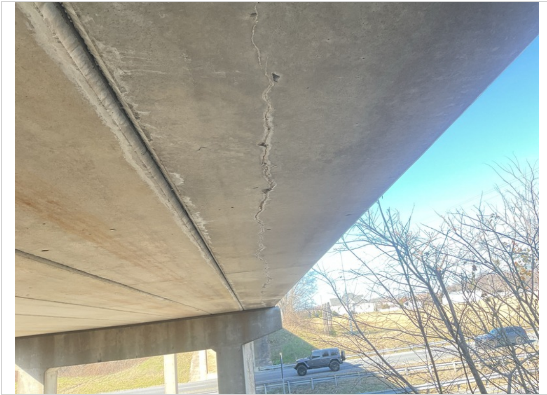
CRACK IN BOTTOM OF BOX BEAM "A", SPAN #4
