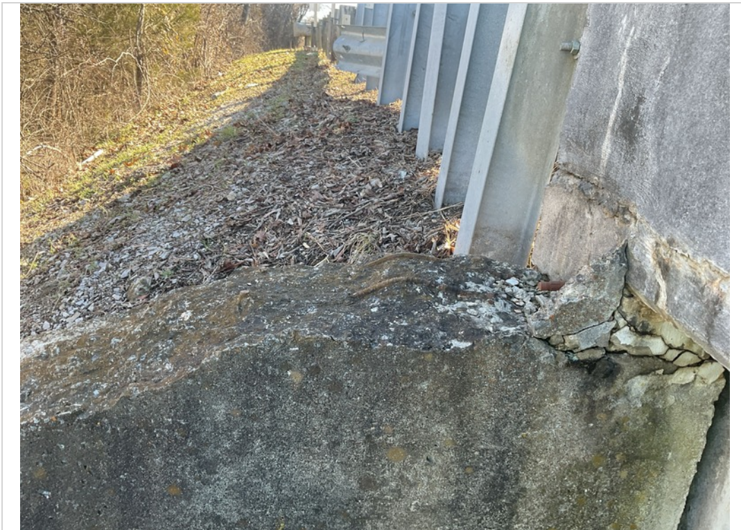
SPALL W/ REBAR IN TOP OF ABUT. #2 LEFT WING
