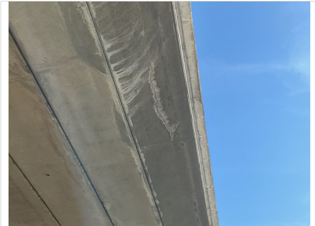
CRACK IN BOTTOM OF BOX BEAM "I", SPAN #2
